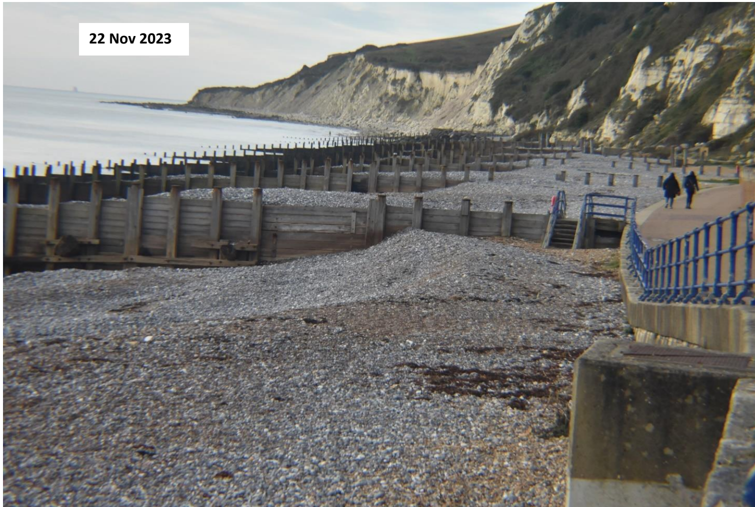
Figure 15: The beach adopts an undulating upper beach profile and the orange-brown ballast is displaced by grey cobbles indicating that the beach is becoming stable with the correct grade of sediment. The larger clasts eventually displace the ballast, further stabilising the beach.
